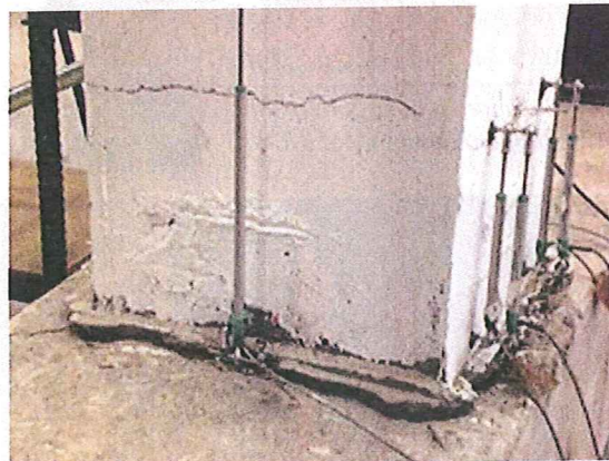
Fig. 11: Slip between jacket and foundation base
